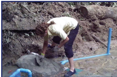
Fort Lewis CO-AMP student Rachel Medina (at left) works to build a water system in Ban NamHom, Laos as part of the Engineers Without Borders program. Rachel's responsibilities included intake for the system at the water source, collecting GPS data and gathering drinking water. "Being a part of this experience has affected my life forever. I think that having the chance to do these projects and build lasting relationships is what really makes sustainability," Medina said.
