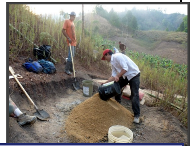
Above, Noah Garcia and a villager mix concrete for the tank, and below, Ashley Garcia cuts bamboo.
